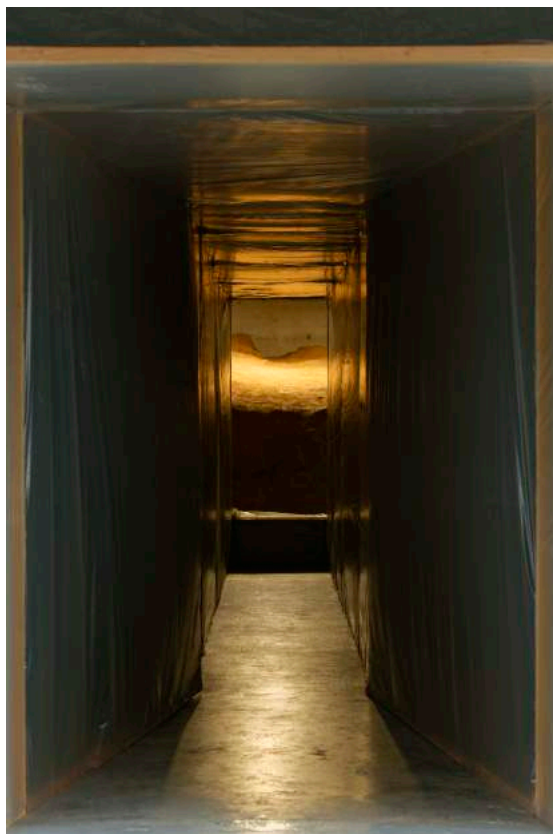
Rebecca Digne, À la hauteur de la terre, 2018 A narrow tunnel leads to the base of the art centre, crawl space voluntarily left to view by architects Aldo Rossi and Xavier Fabre. Photos © Aurélien Mole / CIAP de Vassivière
